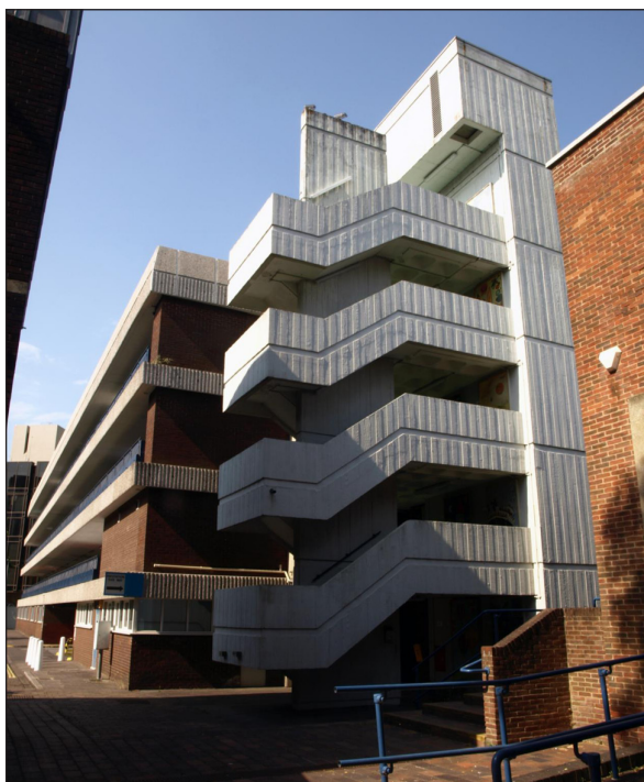
Figure 3: W. D. Worden, Isambard Brunel Car Park, Portsmouth, United Kingdom, Concrete staircase. Photo: Szopinska-Mularz.
